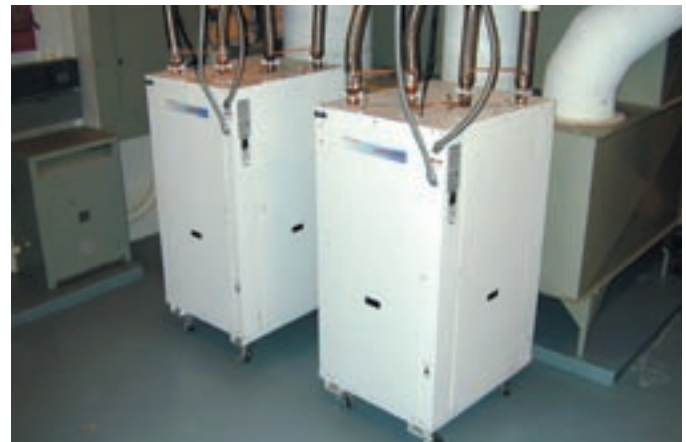
Two 36-ton heat pumps being used for space heating at the College of Southern Idaho.
