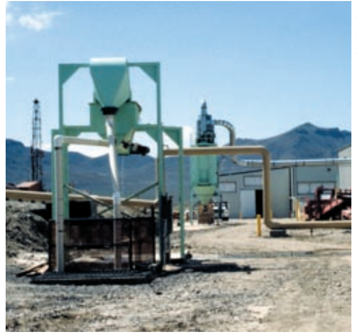
Geothermal energy is ideal for dehydration operations (onions and garlic), as seen in Empire, Nevada.
